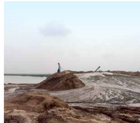
A sand mining project in the Lake Nokoué basin as one of the many development activities in the area.
