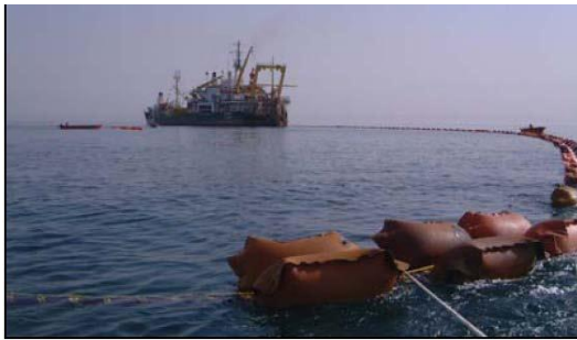
Figure 15: Cable with cable floats
