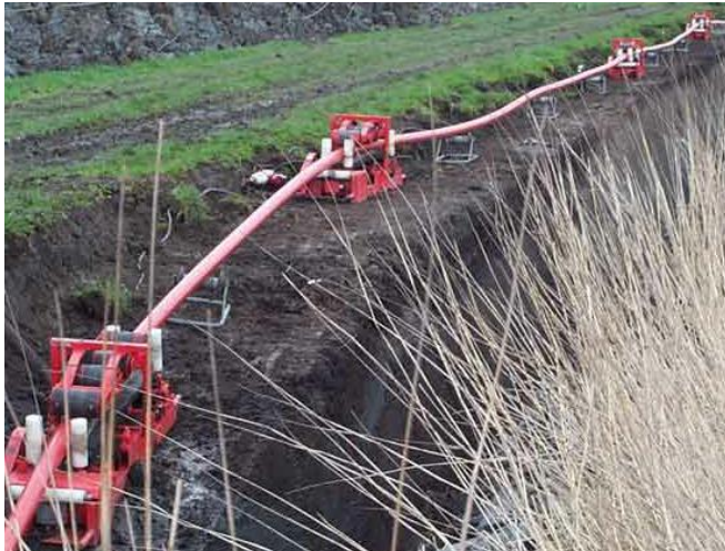
Figure 8: Typical cable tensioners
