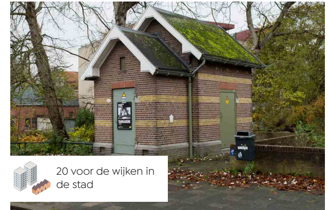
MS-MS station (3-23kV)
